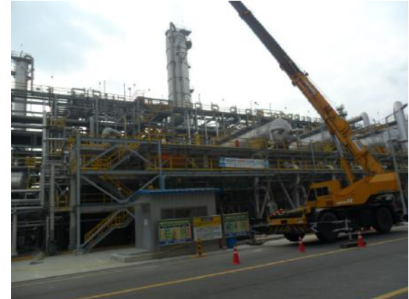
➤ HYUNDAI OIL BANK Alkylation Plant ▶ 18
