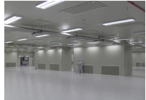
➤ LG DISPLAY P9 Facility ▶ 13
