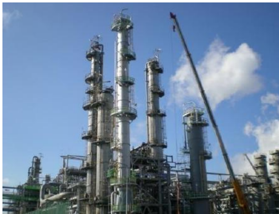
➤ LOTTE CHEMICAL NCC Plant ▶ 35
