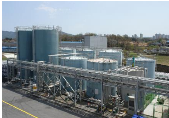
➤ SANNOPKO Rust Preventing Plant ▶ 10
