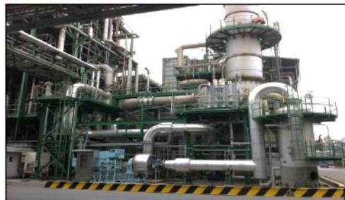
➤ Samsung Fine Chemical MVR Project
