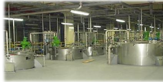
◀ Chemical Supply System in Korea♪
