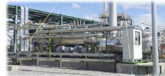
◀ Hot Oil Unit in Gas Separation Plant in Thailand♪
